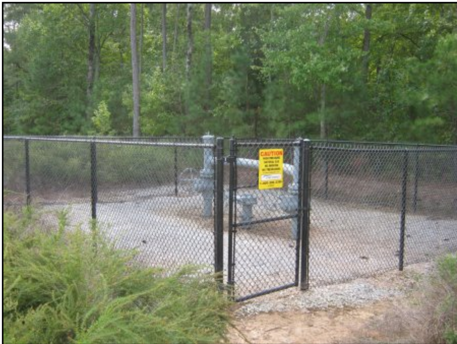
View of PSNC Energy natural gas pipeline utility on the northeastern boundary of the Property.
