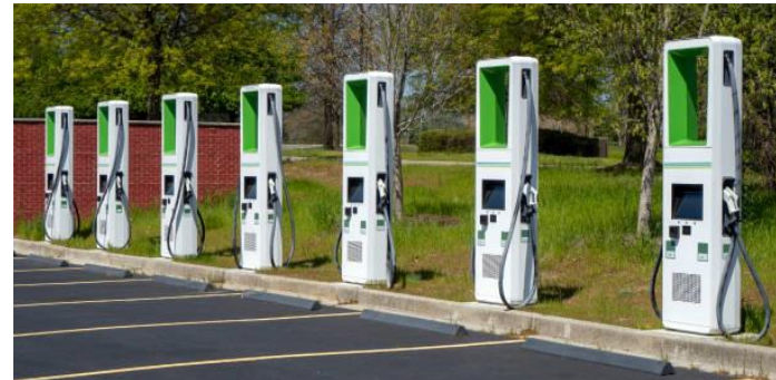
EV Charging Stations
