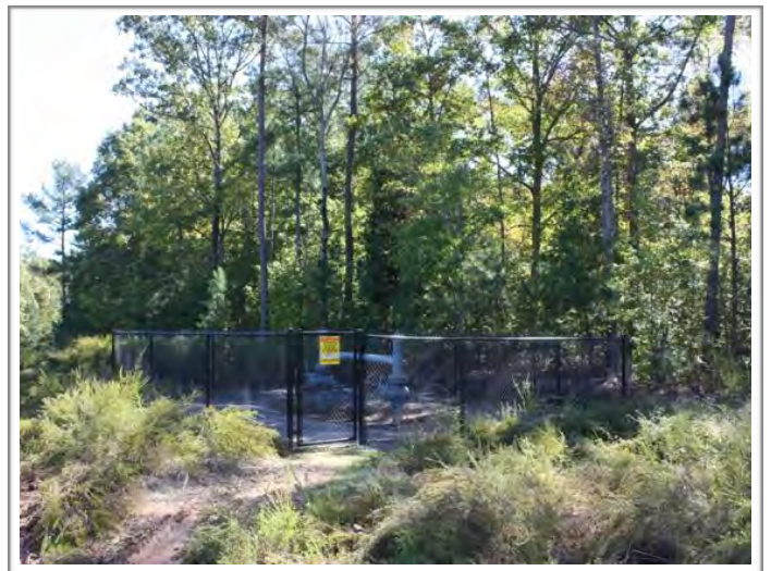
Natural Gas Valve Near North Boundary
